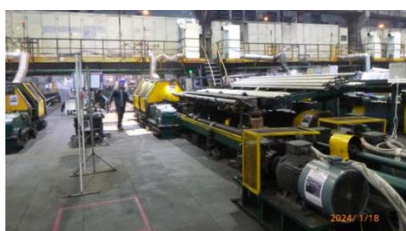
44. Section of cold rolling mills of TDS
